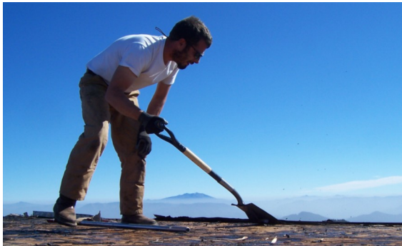
A Kunert employee works on the roof of Fairview Lookout against a backdrop of distant hills and mountains.
