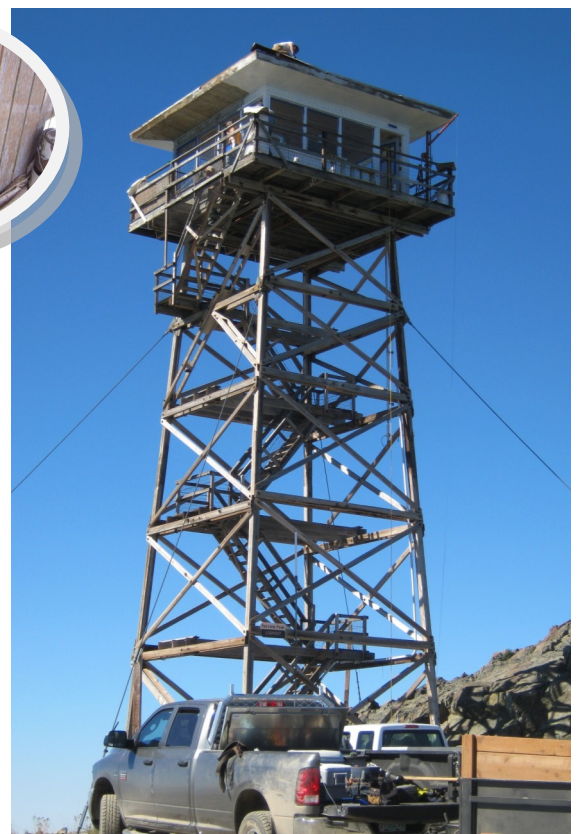
Painting at Fairview Lookout. The insert shows how worn the old paint had become.
